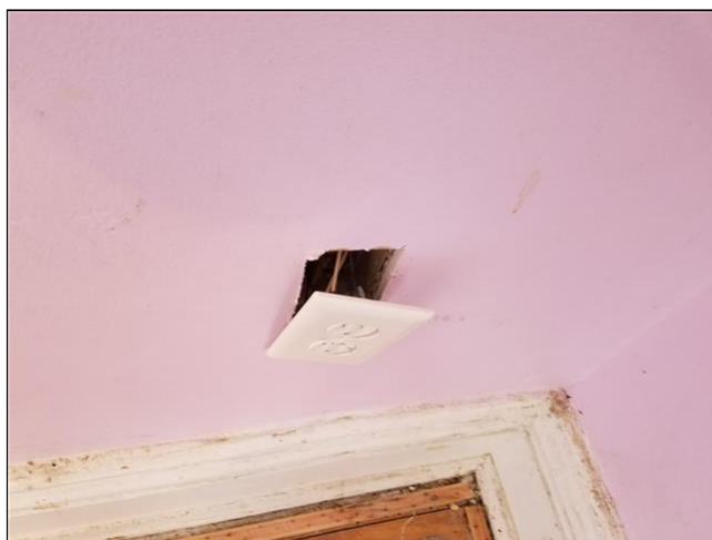
6.3 Item 6(Picture) Example of loose receptacle in front bedroom
