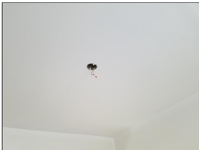
6.3 Item 7(Picture) Exposed wires, missing light Front exterior light post has loose components.
