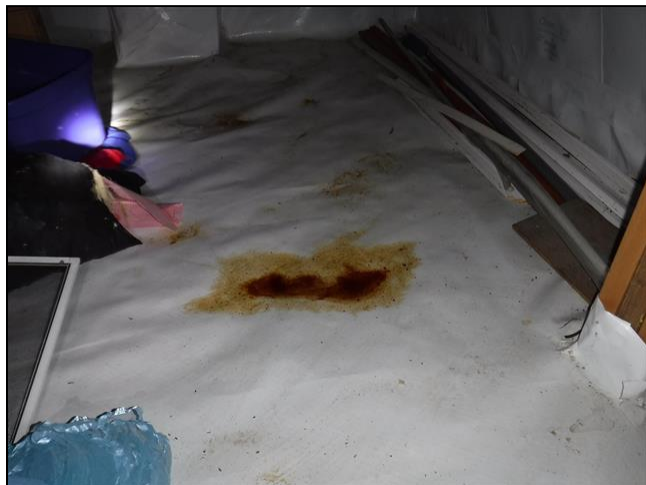
4.0 Item 4(Picture) Small puddle in basement
