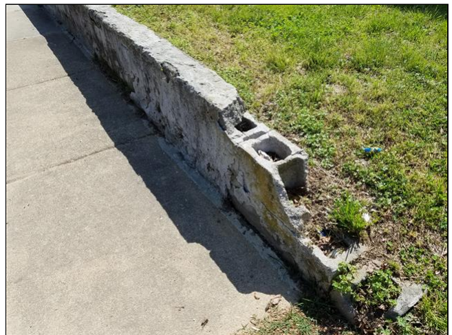
2.4 Item 6(Picture) Front retaining wall damage
