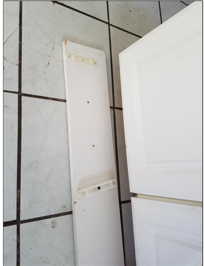
3.4 Item 2(Picture) Cabinet door fell off
