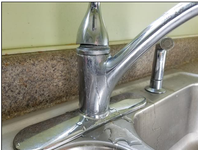
5.0 Item 3(Picture) Leaking fixture (1) Loose condensate drain at left side.
