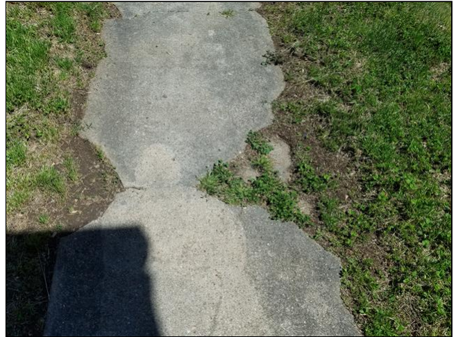
2.4 Item 2(Picture) Example of sidewalk damage
