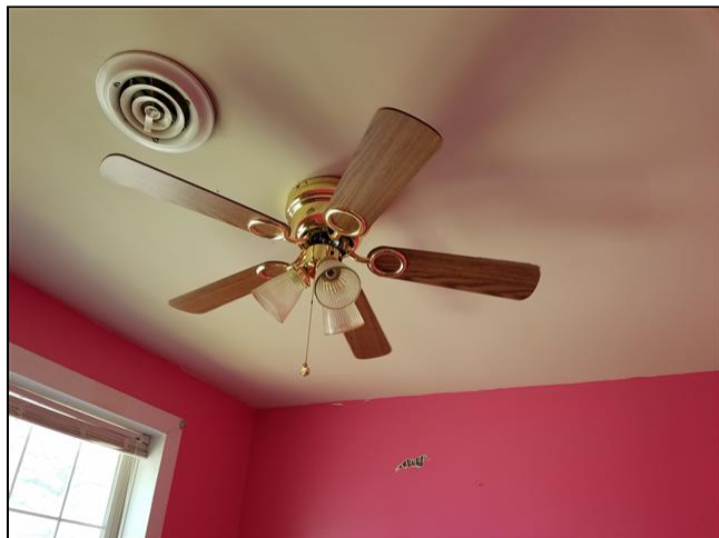
6.3 Item 3(Picture) Fan excessively wobbles
