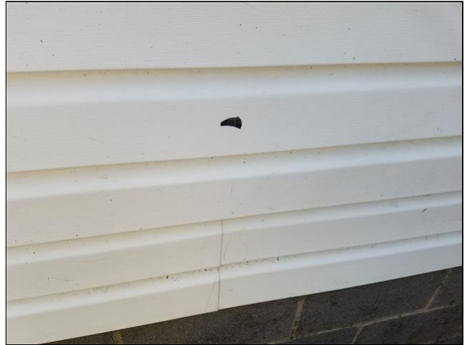
2.0 Item 2(Picture) Example of siding damage, at rear
