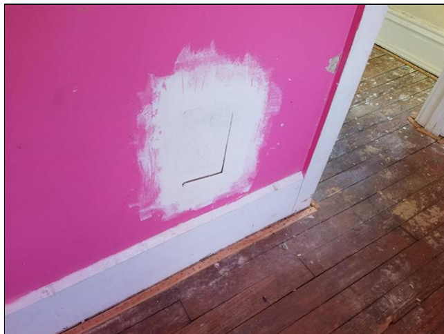
3.1 Item 2(Picture) Example of wall damage
