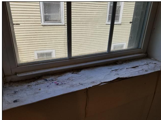
3.1 Item 1(Picture) Water damage at bathroom window area
