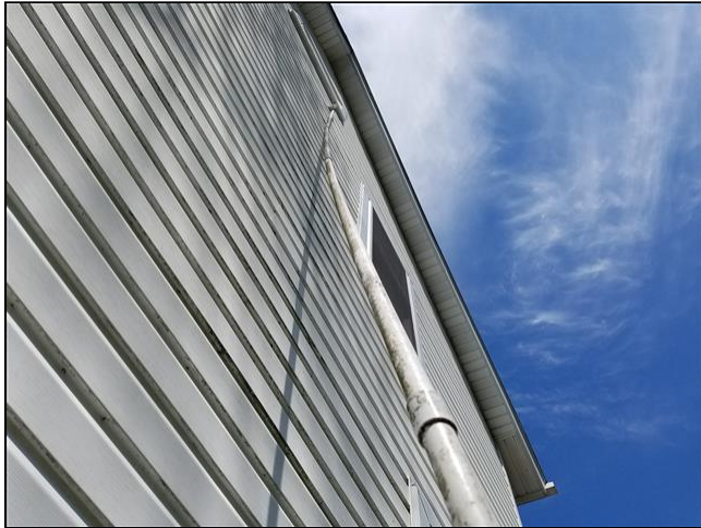
5.0 Item 1(Picture) Loose drain at side
