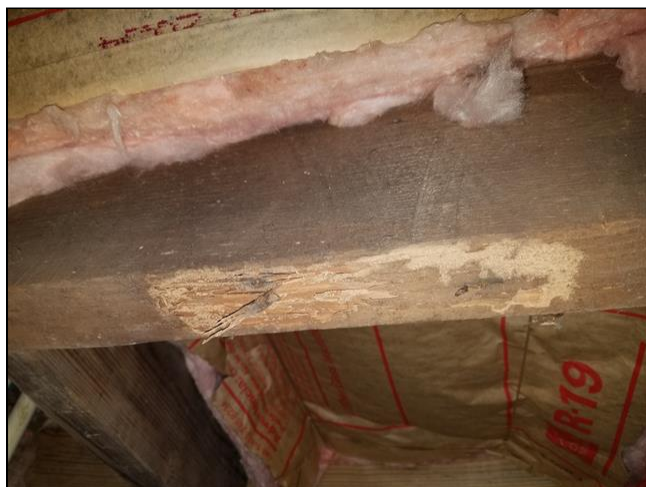
4.1 Item 1(Picture) Appearance of insect damaged joist at rear of basement
