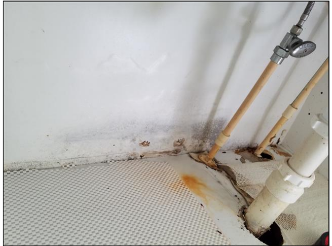
5.0 Item 2(Picture) Mold under kitchen sink
