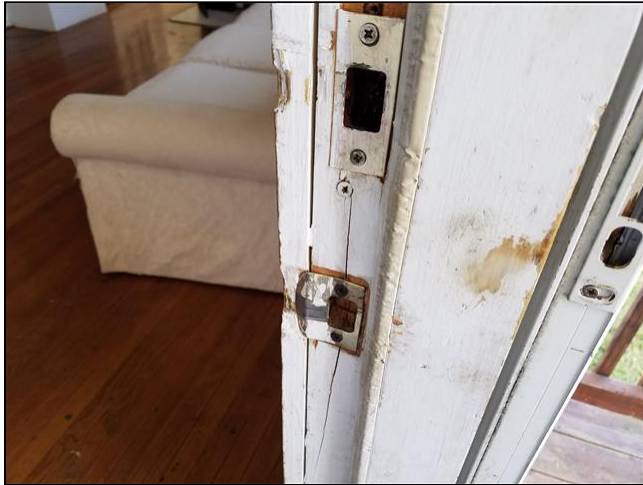
2.1 Item 1(Picture) Cracked door frame
