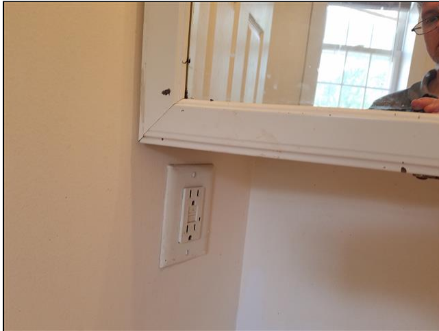
3.4 Item 1(Picture) Cabinet door can't close
