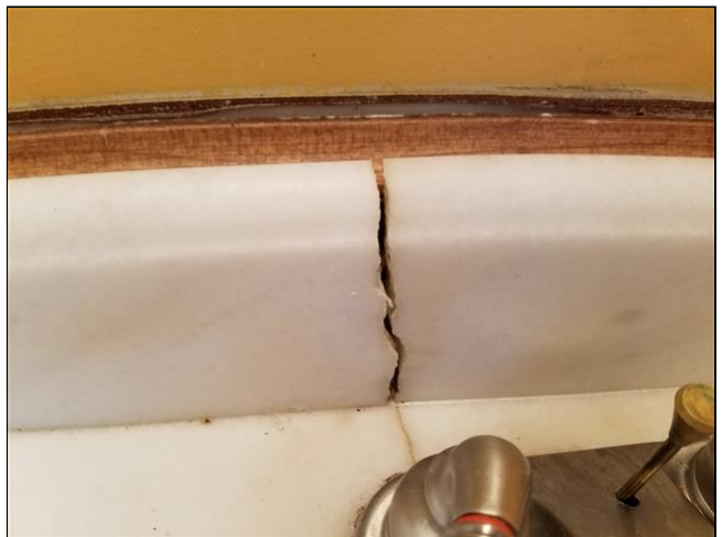
5.0 Item 4(Picture) Cracked backsplash
