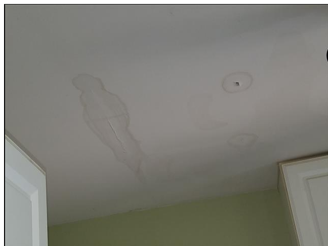
3.0 Item 1(Picture) Moisture stains in kitchen ceiling
