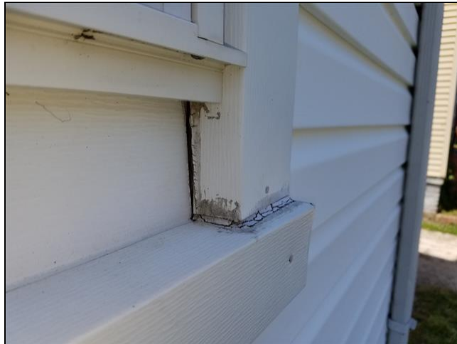
2.5 Item 1(Picture) Example of cracked caulk at window
