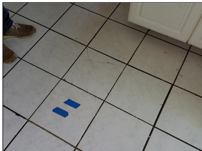
3.2 Item 1(Picture) Damaged tiles in kitchen
