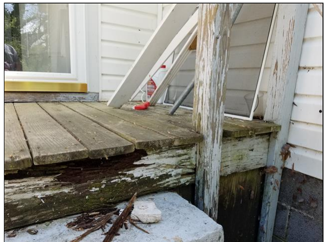
2.4 Item 4(Picture) Example of of damage and missing pickets at rear stairs areas
