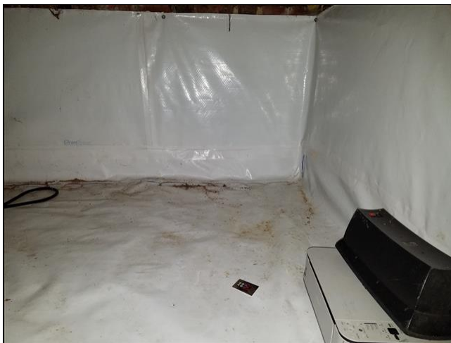
4.0 Item 3(Picture) Covered areas of foundation not inspected
