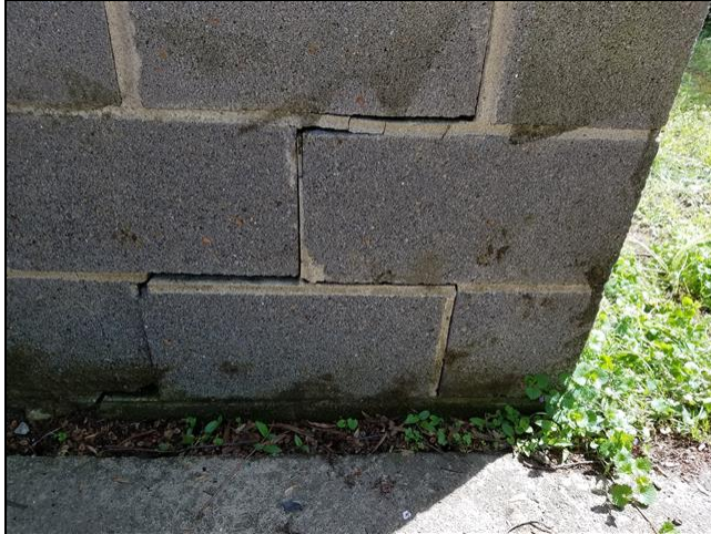
4.0 Item 1(Picture) Foundation crack at rear corner
