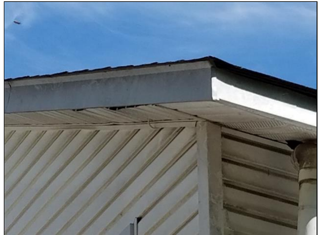
2.5 Item 2(Picture) Loose soffit at rear
