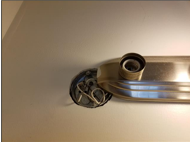
6.2 Item 1(Picture) Uncovered wires in bathroom Uncovered wires in bathroom.
