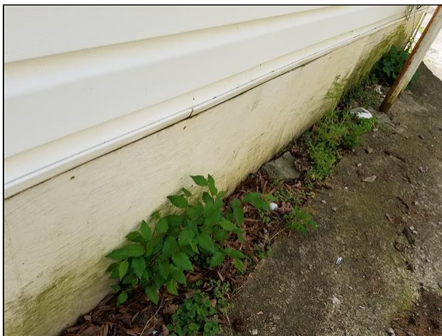
2.0 Item 3(Picture) Wood siding in ground contact Minor siding damages seen.
