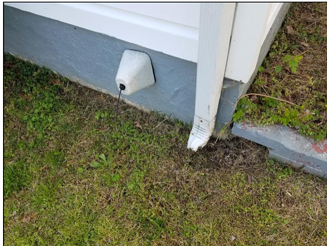
1.2 Item 1(Picture) Bent downspout, winterized hose bib, missing splashblock
