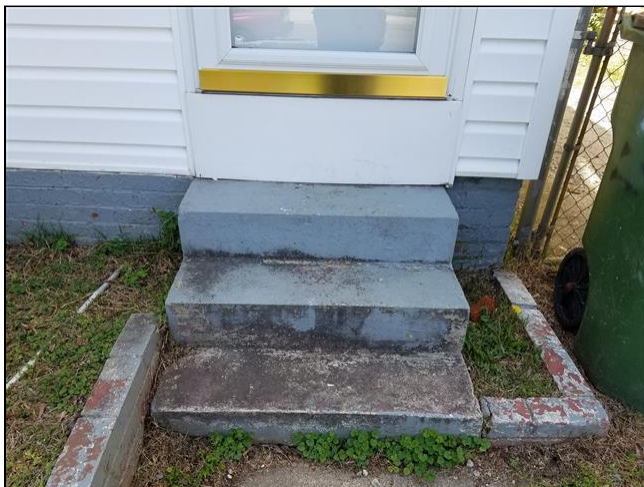
2.4 Item 5(Picture) Missing step height, uneven step height
