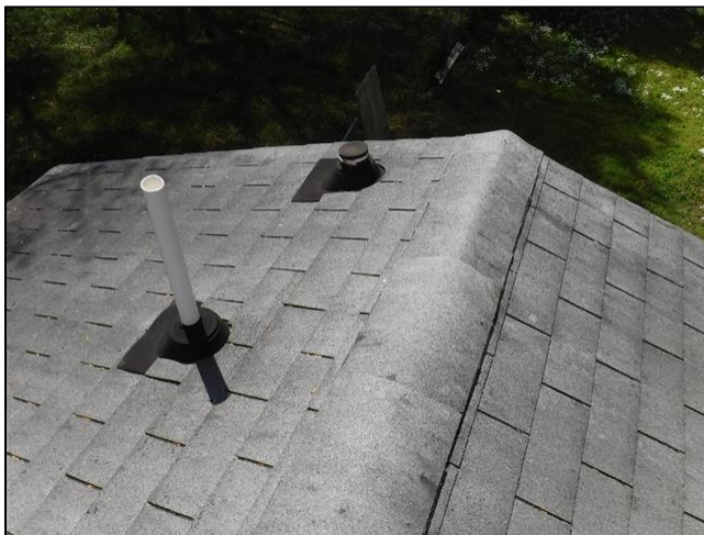
1.0 Item 3(Picture) Example of old shingles
