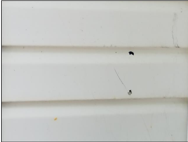
2.0 Item 1(Picture) Example of minor siding damage at rear
