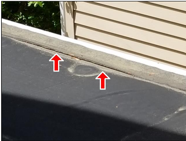
1.0 Item 1(Picture) Example of loose roof seam
