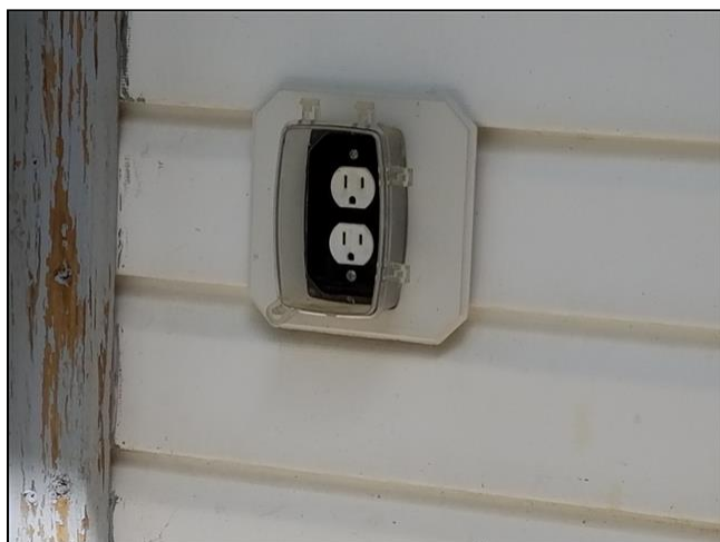
6.3 Item 5(Picture) Cover missing at rear
