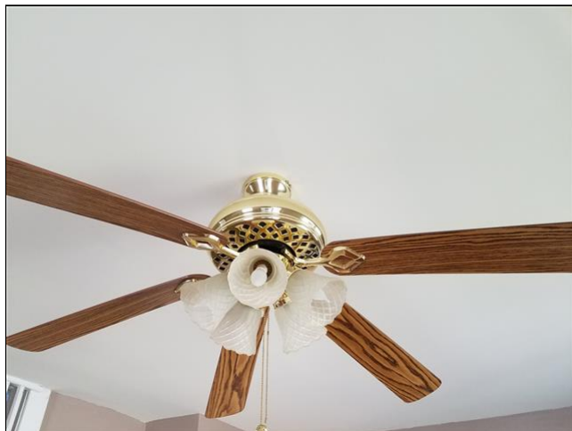
6.3 Item 4(Picture) Missing and drooping blades in living room
