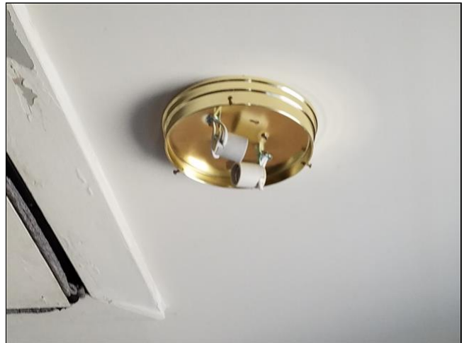
6.3 Item 2(Picture) Example of non functional lights
