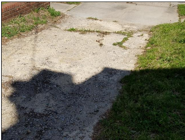
2.4 Item 3(Picture) Deteriorated driveway
