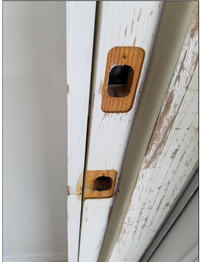
2.1 Item 2(Picture) Strike plates missing
