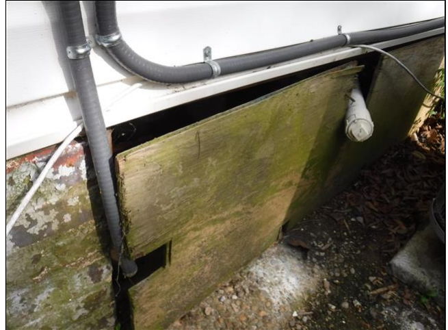
4.0 Item 2(Picture) Removing this crawlspace access panel may damage drain. Crawlspace access isn't readily accessible
