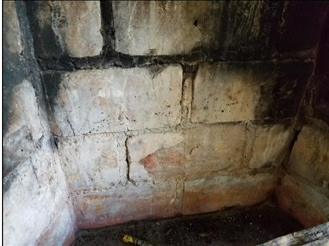
7.4 Item 1(Picture) Deteriorated firebox
