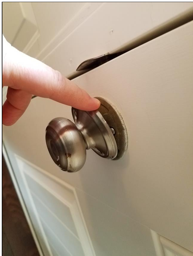
2.1 Item 1(Picture) Loose knob cover Loose cover plate at front and rear door knobs.
