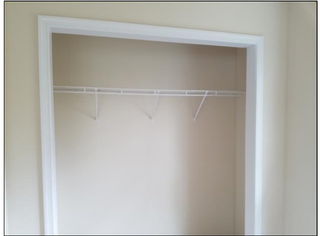
4.5 Item 2(Picture) No closet doors installed at rear bedroom
