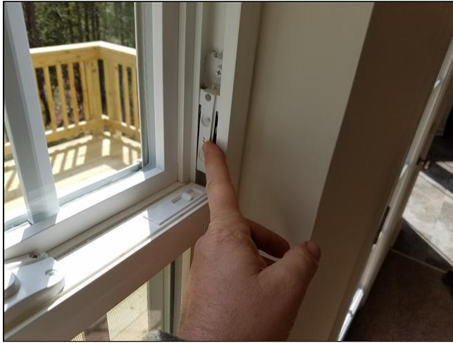
4.6 Item 1(Picture) Family room window needs repair Family room window not functioning properly.
