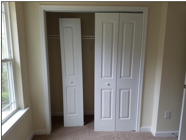
4.5 Item 3(Picture) Closet door not installed, rear bedroom
