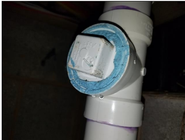
6.0 Item 4(Picture) Close up of leak in crawlspace
