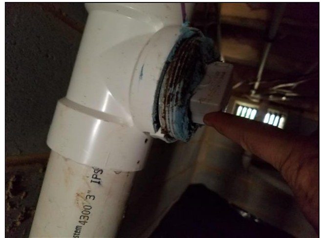
6.0 Item 2(Picture) Cleanout cap area damaged
