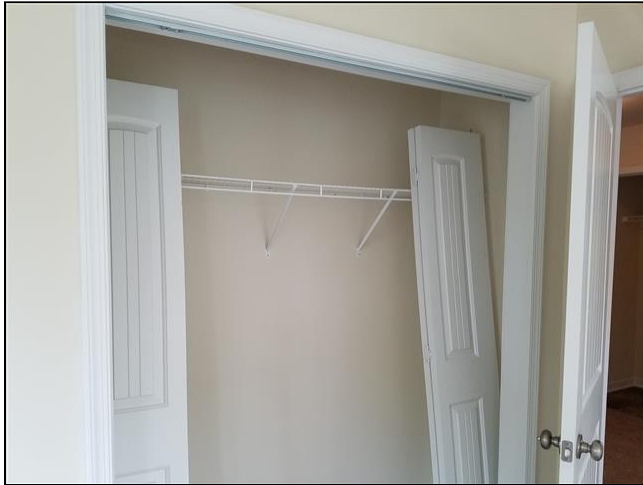
4.5 Item 1(Picture) Closet doors not installed
