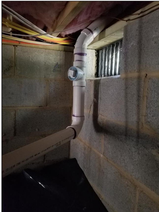
6.0 Item 3(Picture) Leak seen here
