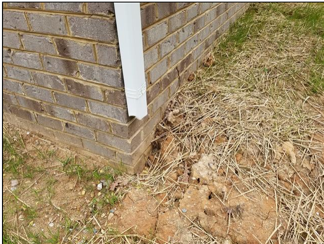
1.2 Item 1(Picture) Downspout elbow missing
