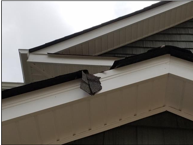
1.0 Item 1(Picture) Shingle damage at front
