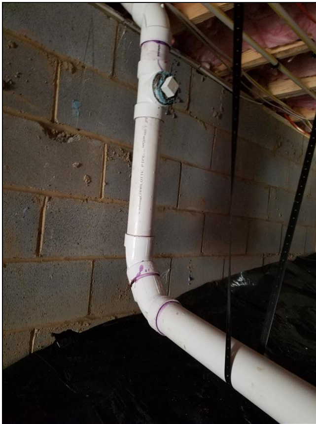
6.0 Item 1(Picture) Leak seen at this drain area
