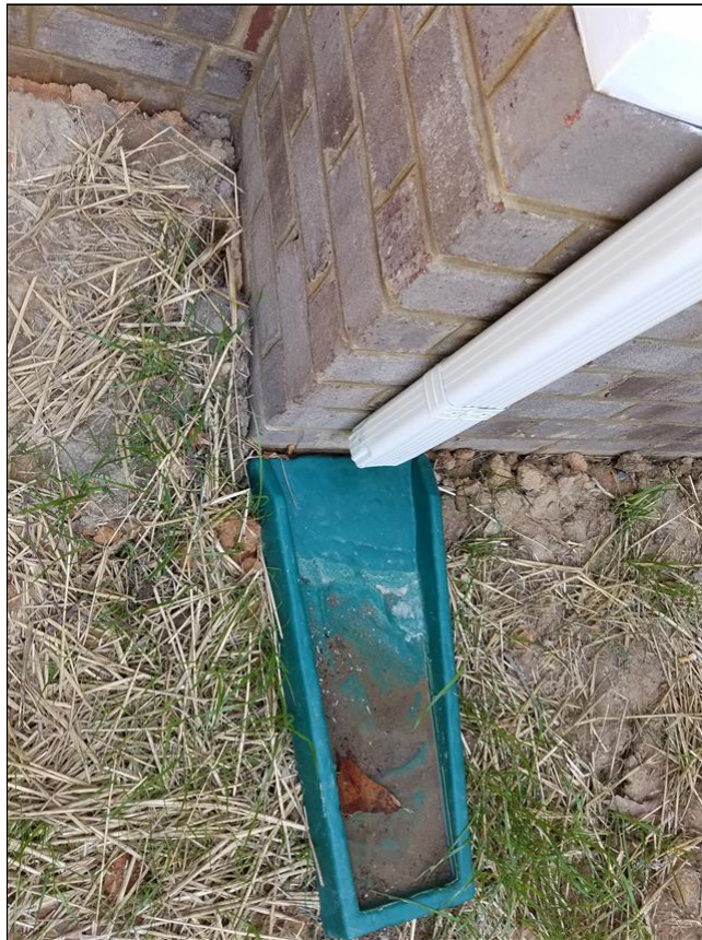
1.2 Item 2(Picture) Missing elbow, splashblock is backwards
