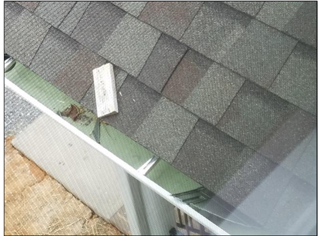
1.0 Item 2(Picture) Construction debris on roof and gutter
