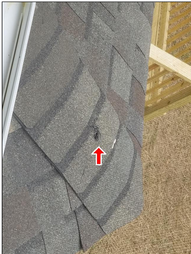
1.0 Item 3(Picture) Shingle damage at rear bumper out
