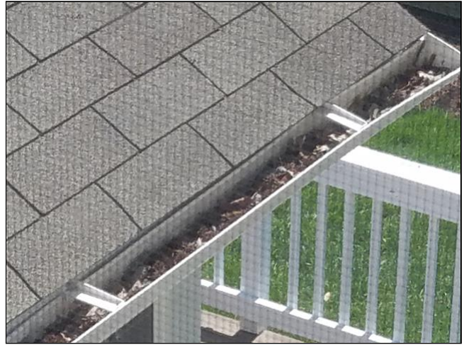
1.2 Item 2(Picture) Gutter cleaning recommended
