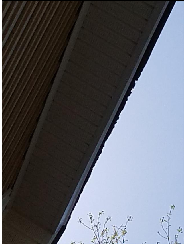
1.0 Item 1(Picture) Example of shingle damage at gable
