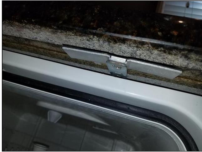
10.0 Item 1(Picture) Loose bracket at dishwasher Loose bracket at top of dishwasher.
