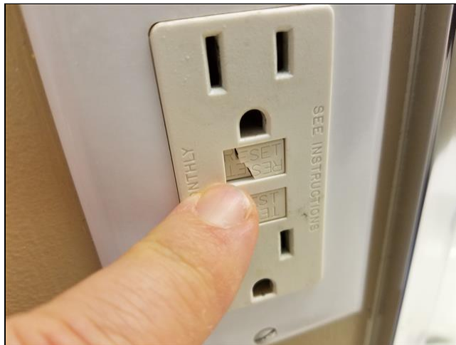
7.3 Item 1(Picture) GFCI damaged in master bathroom
