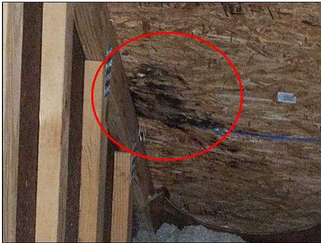
5.3 Item 1(Picture) Sheathing stains and damage
