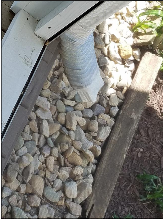
1.2 Item 1(Picture) Rear downspout too short
