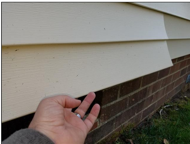
2.0 Item 3(Picture) Example of loose siding at right side
