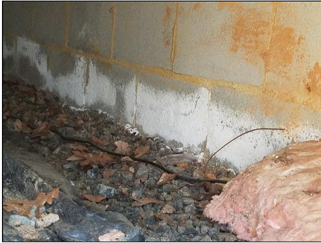
5.0 Item 1(Picture) Example of efflorescence at foundation
