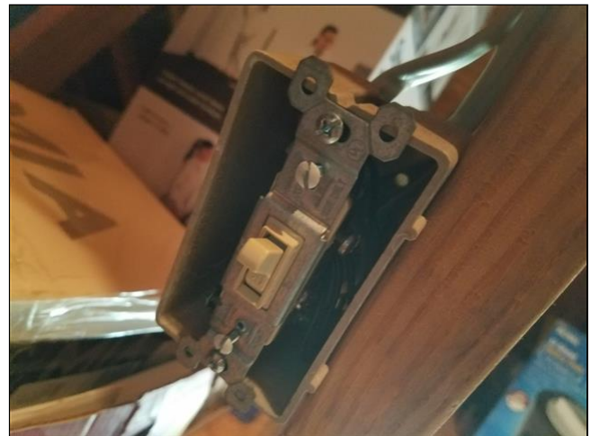
7.3 Item 2(Picture) Switch cover missing in attic
