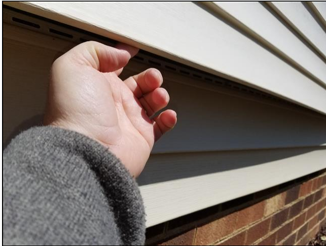
2.0 Item 1(Picture) Example of loose siding at rear
