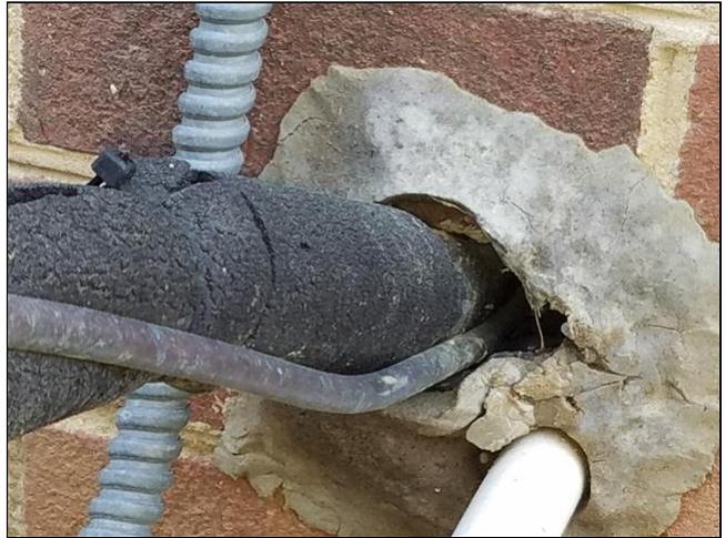
2.0 Item 2(Picture) Seal exterior openings as needed, this is at suction line
