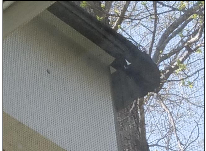
1.0 Item 2(Picture) Example of shingle damage at rear corner
